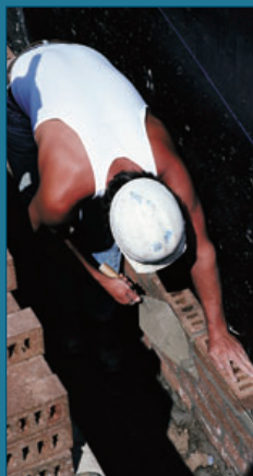
figure qc.5 After the hard work of laying the bricks is done, excess mortar is removed using a brick cleaner with hydrochloric acid as the main ingredient.
