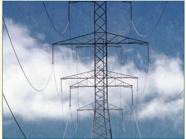
figure es.9 The national electricity grid allows electricity to be produced in remote areas near coal mines and then supplied to cities using high voltage power lines.
